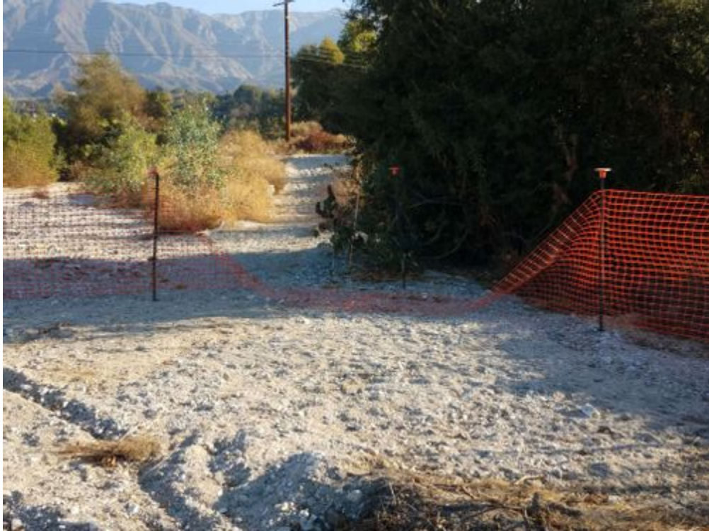
photo_1-20201113_damaged fencing at NE corner_facing N.jpg -118.17081 34.19413
